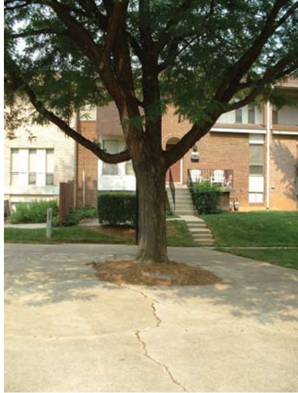
Figure 16. Tree roots cause adjacent pavement to crack.
