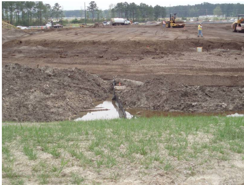
Figure 4. Mass clearing, grading, and removal of topsoil at a construction site (Photo by Center for Watershed Protection)
